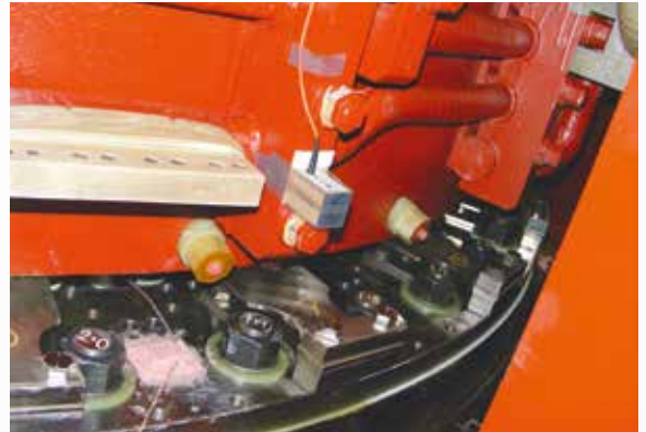
Installation of optical vibration sensors on a power generator
