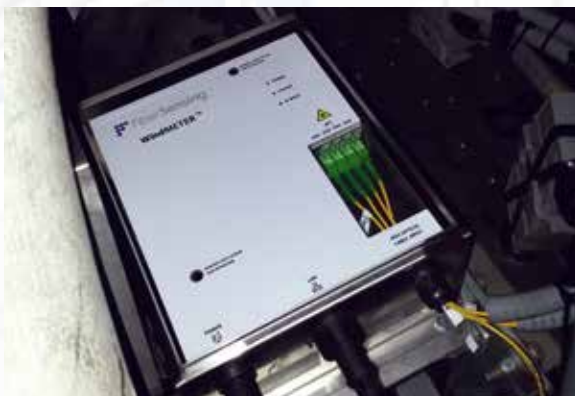
WindMETER interrogator under operation in wind turbine
