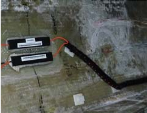
Fig. 2.8 Cable protected with corrugated tubes
