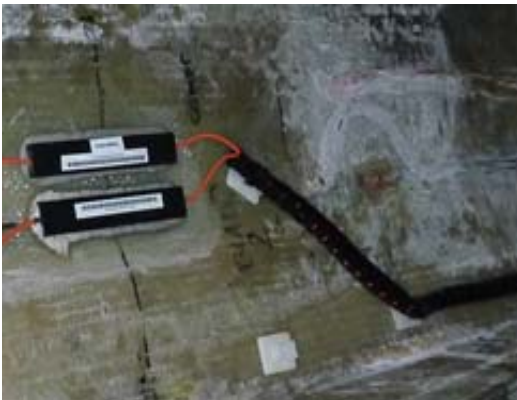
Fig. 2.3 Cable protected with corrugated tubes
