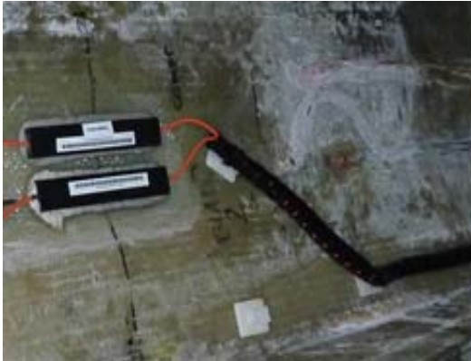
Fig. 3.12 Cable protected with corrugated tubes
