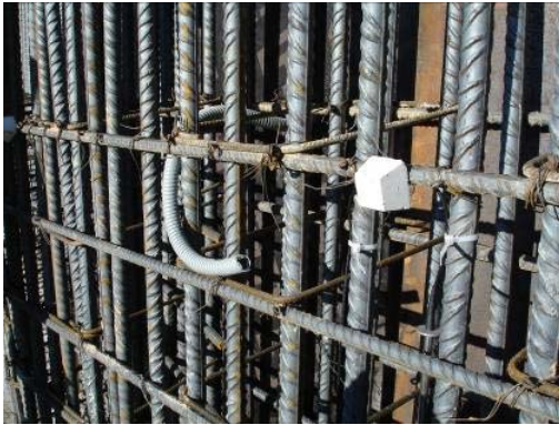
Fig. 2.1 Protection tube from the cable collection point to the sensor installation area
